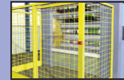
Guard door locked. Operator selects access to machine via selector switch. Machine goes into Safe Limited Speed with Safe Direction mode.
